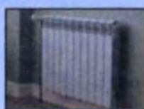
9 radiator (part of a central heating system)
